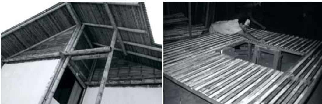
Fig. E.5: One of the 1987 prototypes of the National Bamboo Project (NBP) in Costa Rica. Fig. E.6: A panel factory in Costa Rica.
