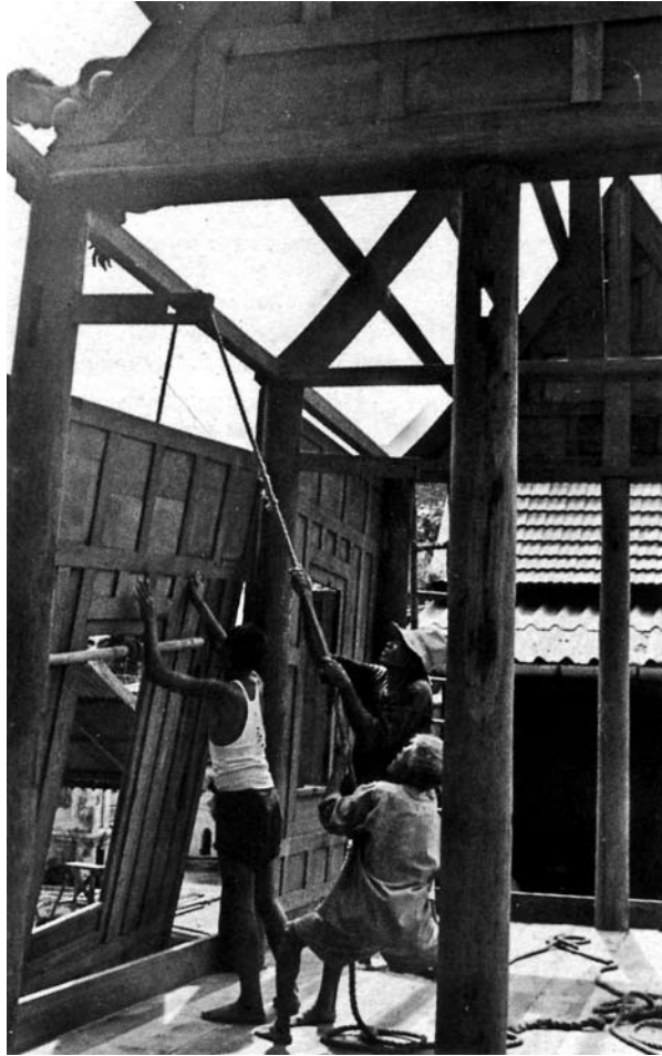
Team work of hoisting a wall panel during a house construction process in Thailand (shown to present how walls of houses in South East Asia are generally light and non load-bearing) / Photo: Dorothy Pelzer Collection, courtesy of ISEAS, Singapore / Source: Roxana Waterson. 1997. The Living House, p. 75
