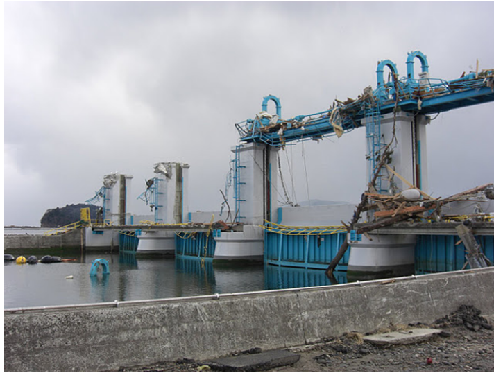
Figure 2: Damaged floodgate at Minamisanriku
