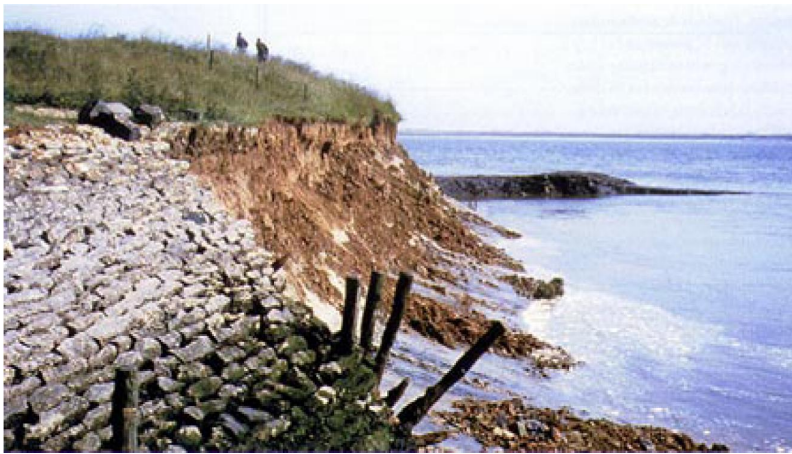
Figure 10. Near failure of a dike due to flow slide
