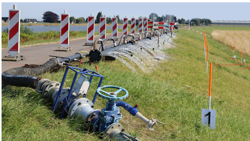
Figure 6.1: Example of proof loading of dikes. Photo courtesy of Michiel van der Ruyt / Deltaras
