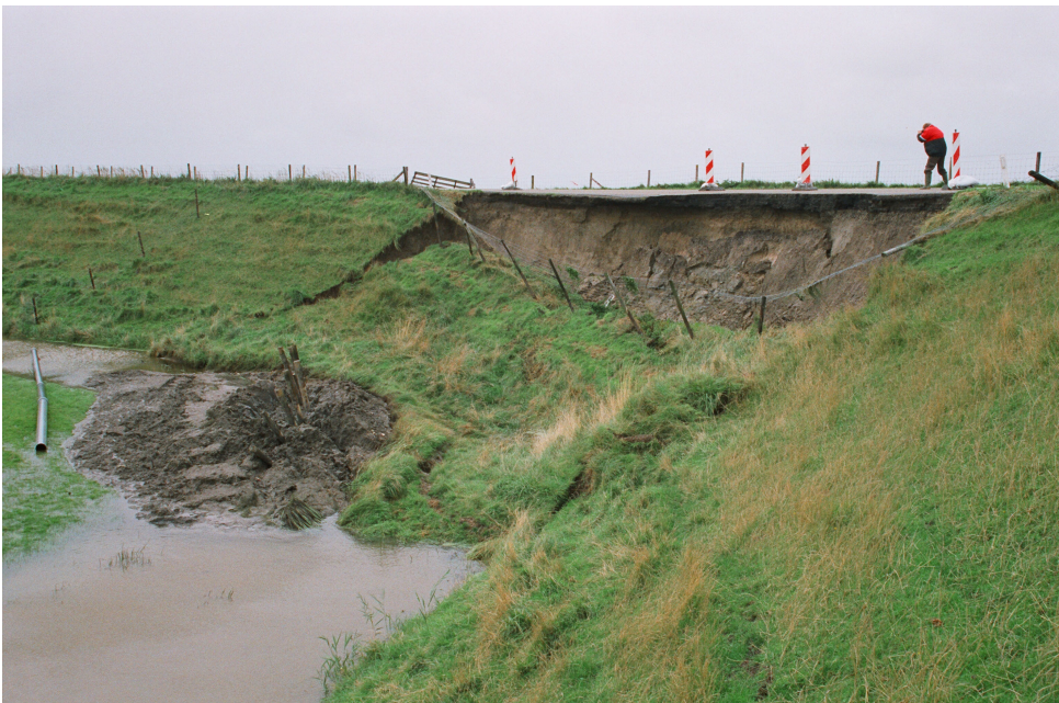
Figure 1.3: Instability of the inner slope of the Westfriese Zeedijk near Sint Maarten in Noord Holland on 15 September 1994 (source: Deltares Visuals)
