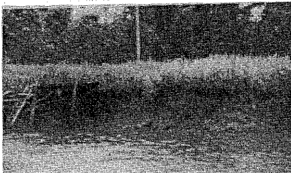
Photo 3: Bank erosion caused by boat waves
