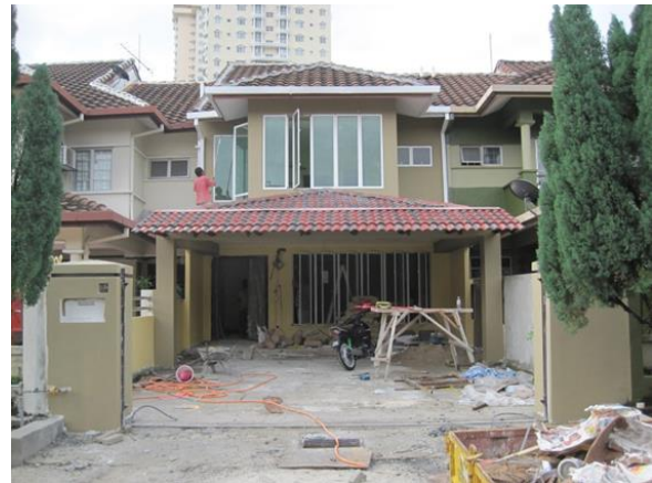
Fig. 4. The renovation has involved a frontal makeover on the façade and changing of windows
