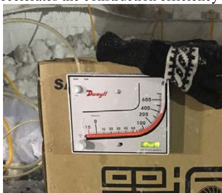
Figure 16: Pressure control equipment
